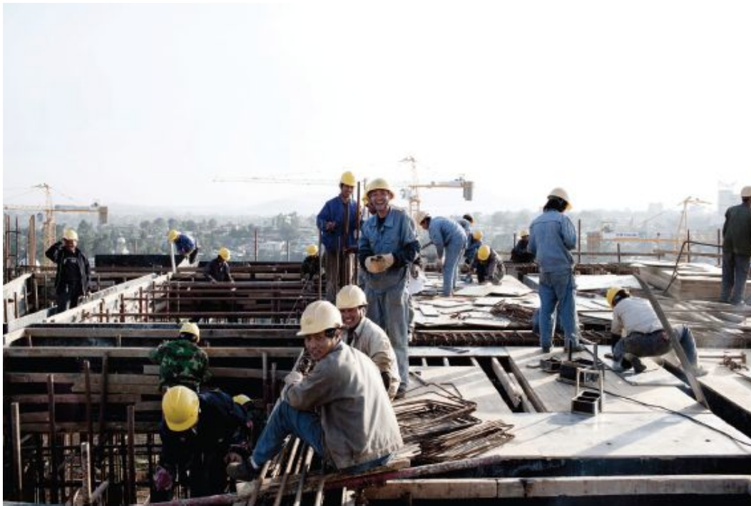
Chinese construction workers build the new African Union Buildings in Addis Ababa, Ethiopia.
